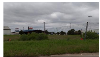
Damaged fence at stormwater catchment Source: Marvin Planning Consultants
