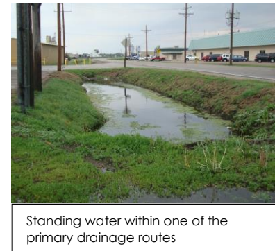
Standing water during a recent rain event
