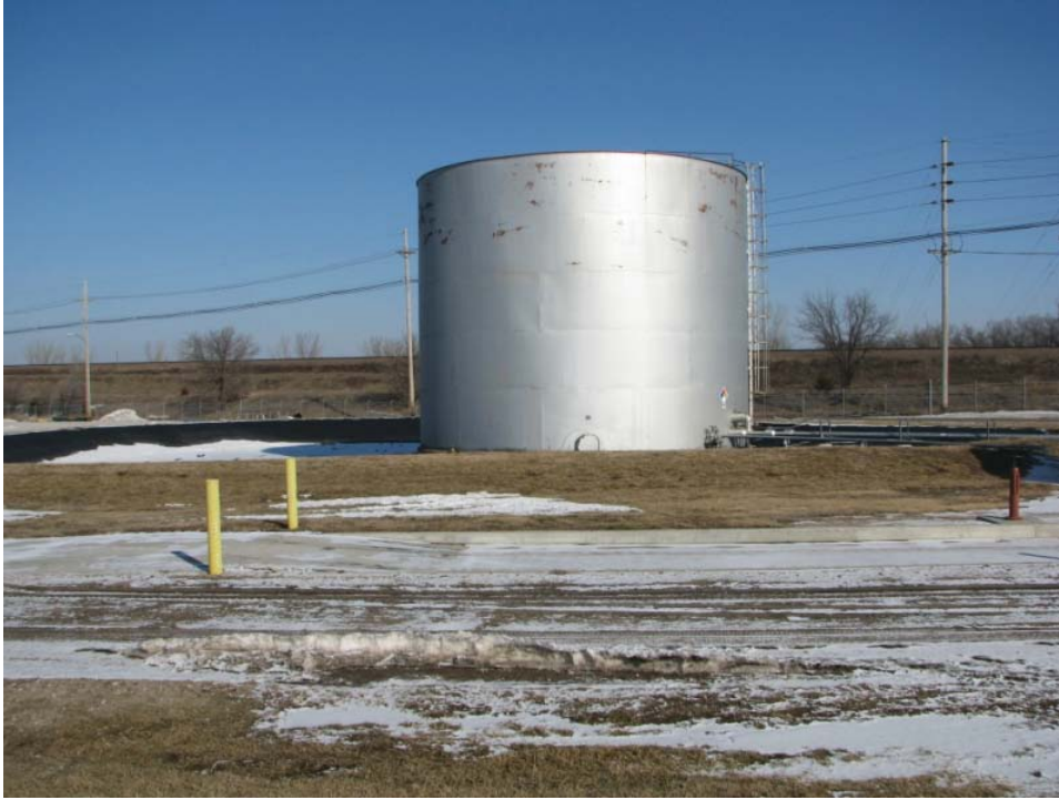
Figure 1 Burdick Station Diesel Fuel Tank Blast and recoat exterior. Lead abatement is assumed to be required.
