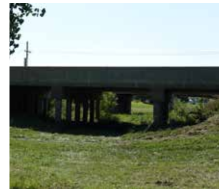
Above: Underpass connection from Stuhr Trail west to new hospital site, a part of a priority trail extension to Cedar Hills Park.
