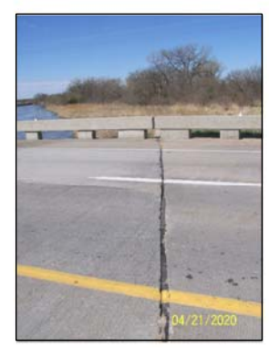
U104504125 - NORTH - END OF FLOOR
