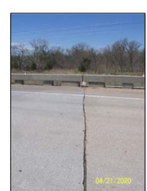
U104504120 - NORTH - END OF FLOOR
