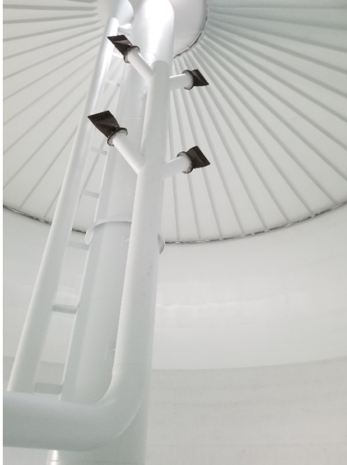
Figure 9 Olson Tower internal mix piping
