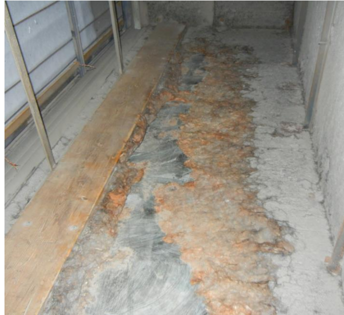
Multi-Zone AHU Interior Condition
