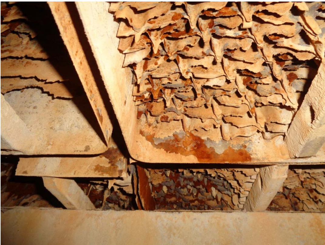
There is substantial loss of element across entire cold end.
