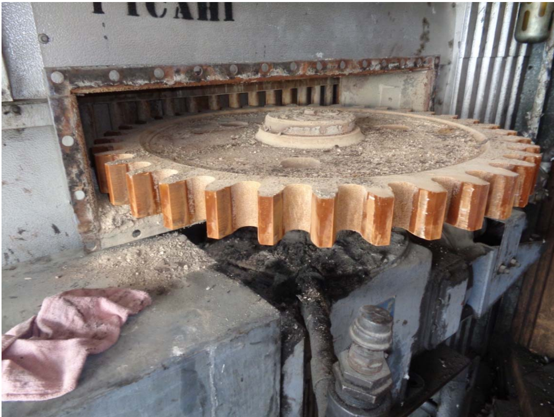
The drive gear shows normal wear and is in good working condition.
