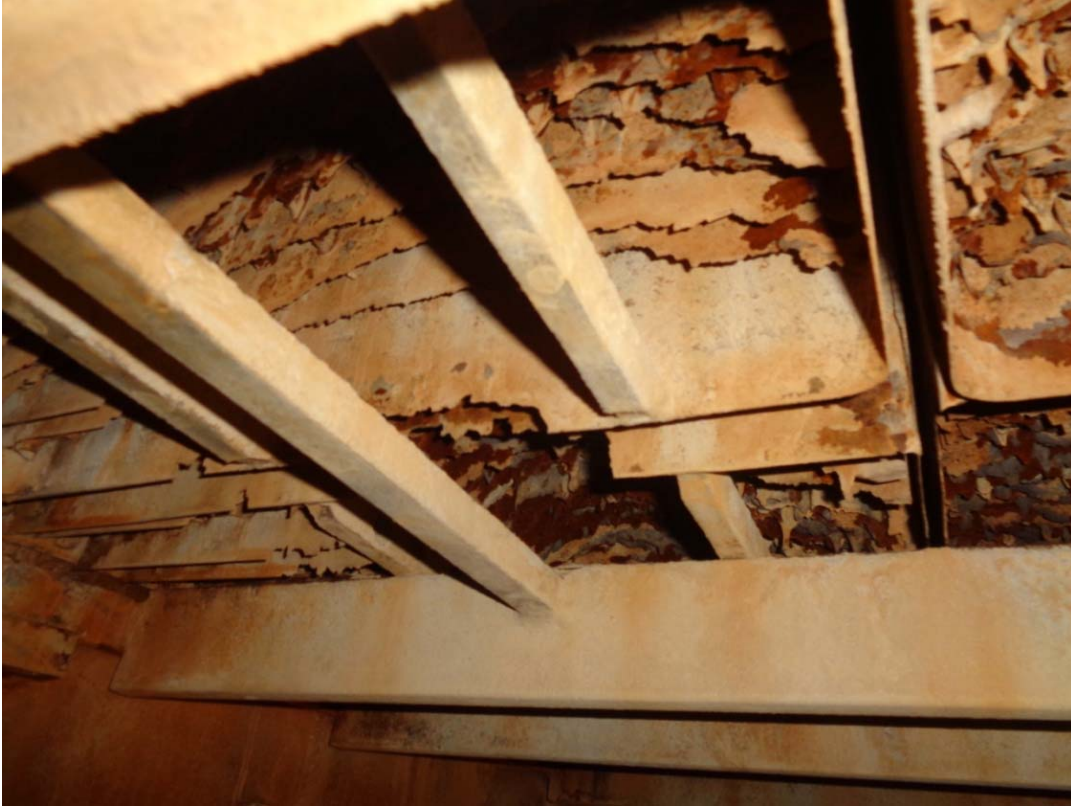
Cold end element is showing significant thinning of the element sheets.
