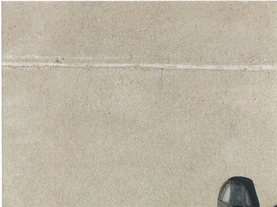
Photo 4 - Typical Hairline Cracks in Topping of Rooftop Level
