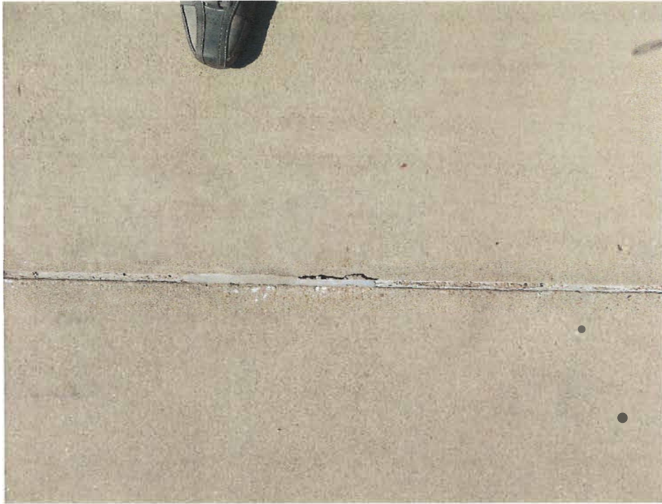
Photo 7 - Example of Poor Seal Joint on Rooftop Level
