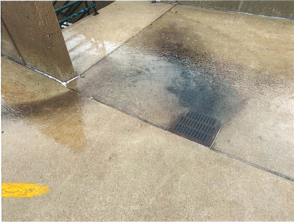
Photo 1 - Plugged Drain at Southwest Corner of Rooftop Level
