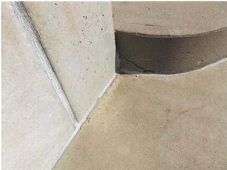
Photo 6 - Spalled Concrete Near Center Railing of Rooftop Level
