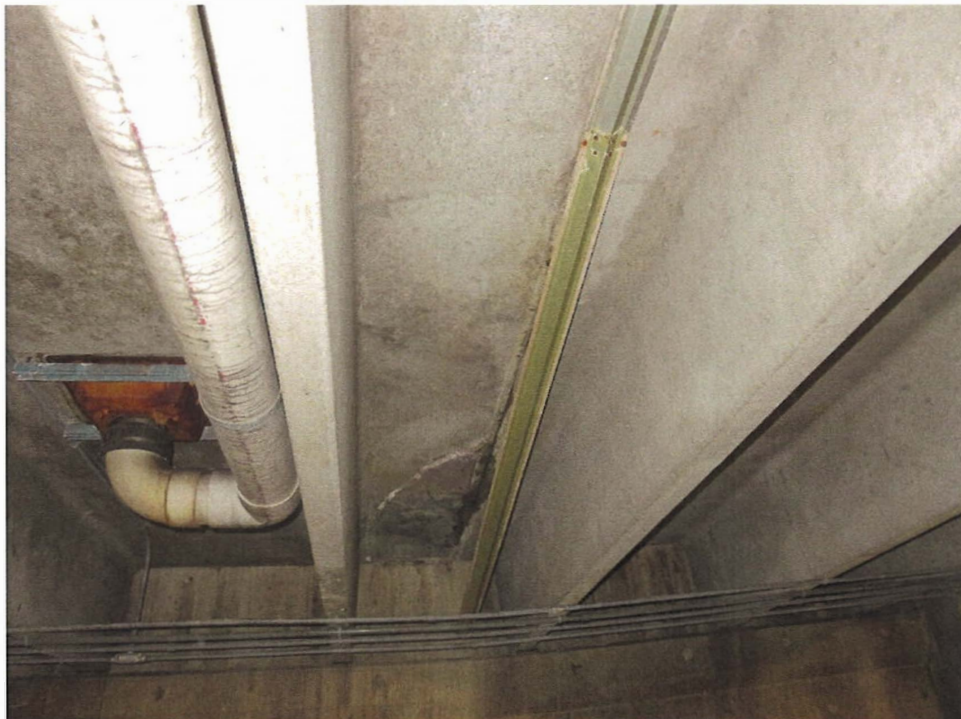
Photo 20 - Partially Fallen Rain Track of Lower Level
