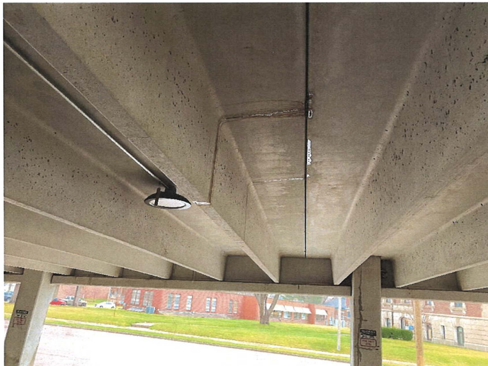
Photo 8 - Example of Rainfall Leak from Rooftop Level
