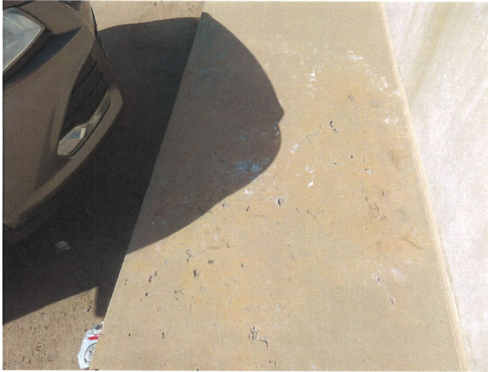
Photo 11 – Surface Deterioration of Sidewalk on North Side of Rooftop Level
