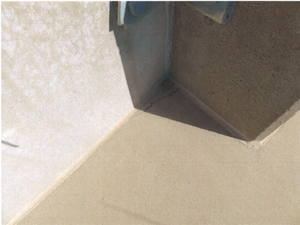
Photo 10 - Example of Spalled Sidewalk on North Side of Rooftop Level
