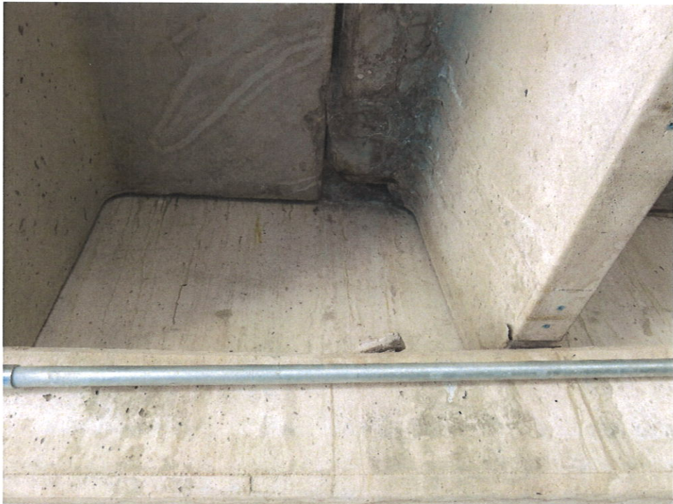
Photo 12 – Spalling of Concrete & Exposed Rebar in Concrete Tee Beam on North End of Main Level
