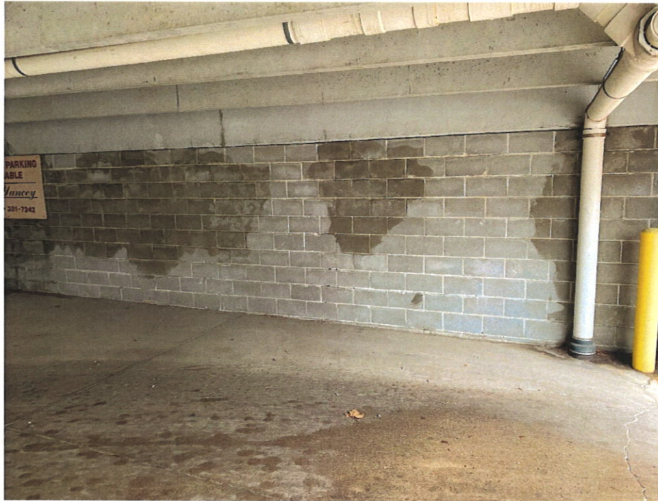
Photo 27 – Evidence of Moisture in CMU During Rainfall Event on East End of Garage
