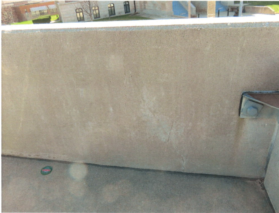
Photo 23 – Diagonal Crack Along South Wall of Rooftop Level
