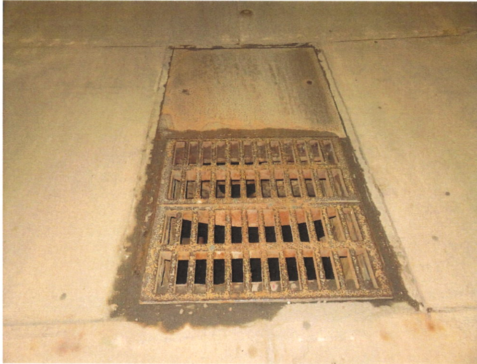
Photo 19 – Large Junction Box w/ Standing Water at Center of Lower Level
