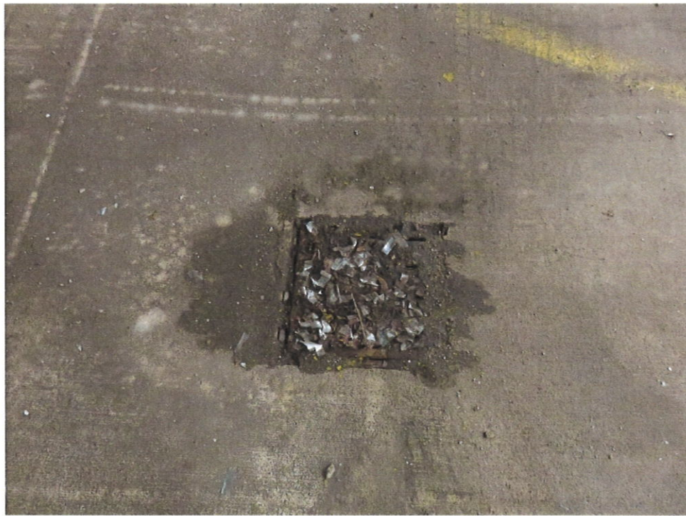
Photo 18 – Typical Floor Drain Clogged with Dirt & Debris Near Center of Lower Level
