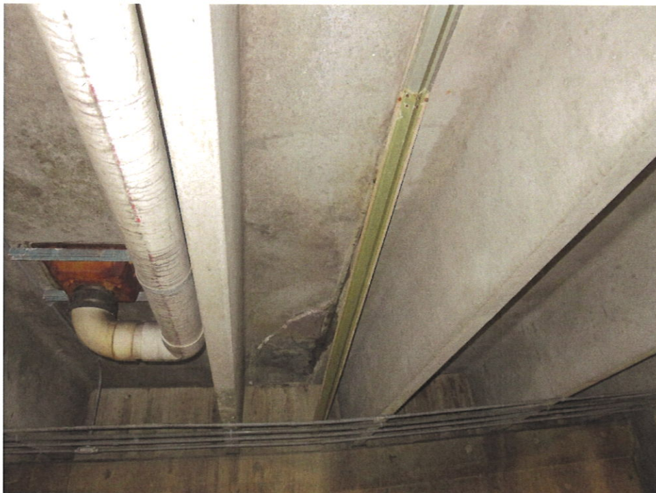
Photo 20 – Partially Fallen Rain Track of Lower Level
