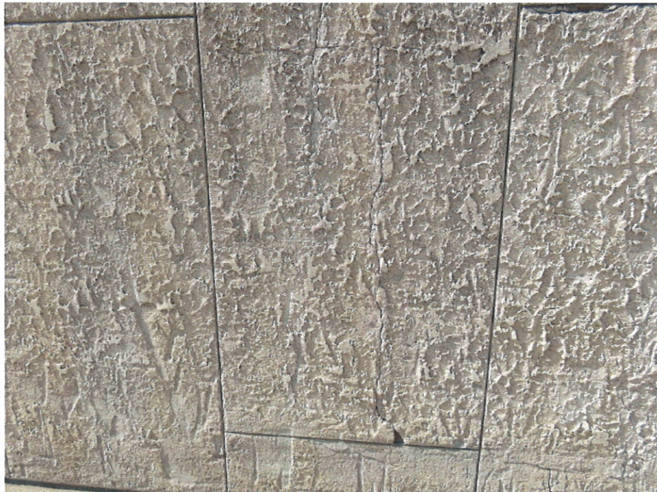
Photo 26 – Example of Significant Cracking in Stucco Finish on East End of Garage
