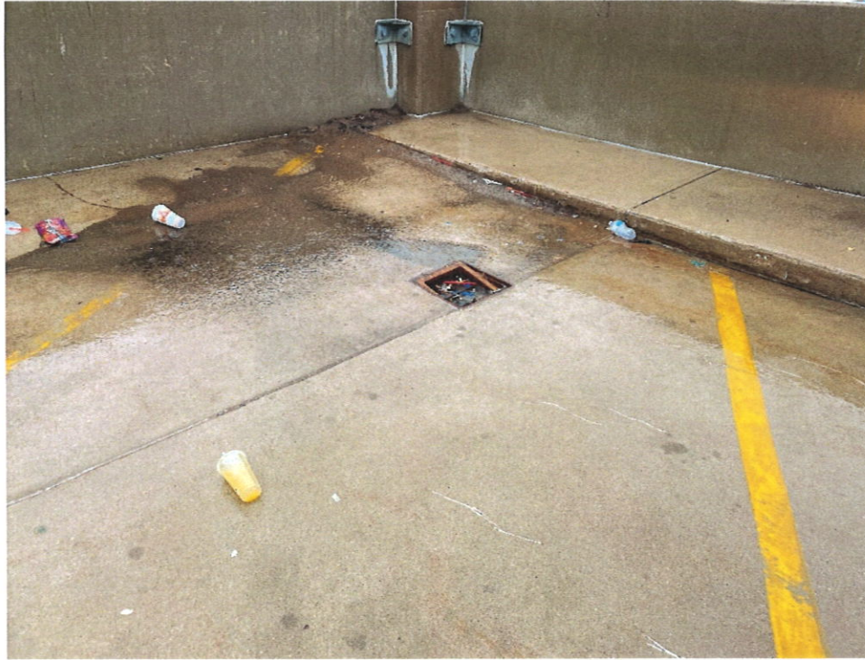
Photo 3 – Ponding and Debris Filled Drain at Southeast Corner of Rooftop Level
