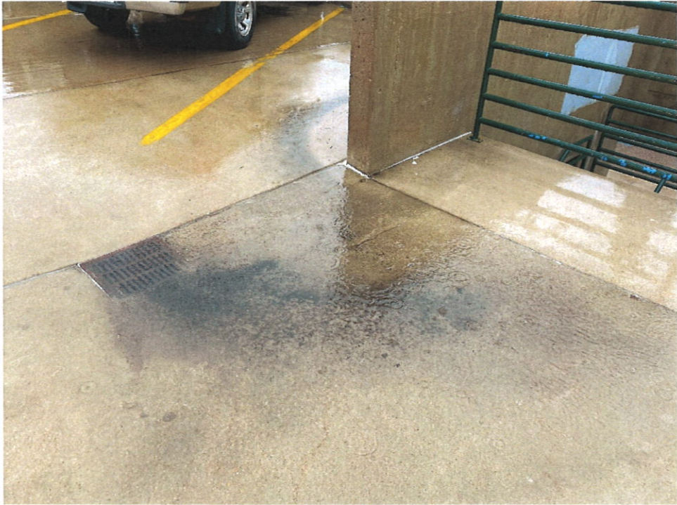
Photo 2 – Rainwater Flowing to Stairwell Due to Plugged Drain
