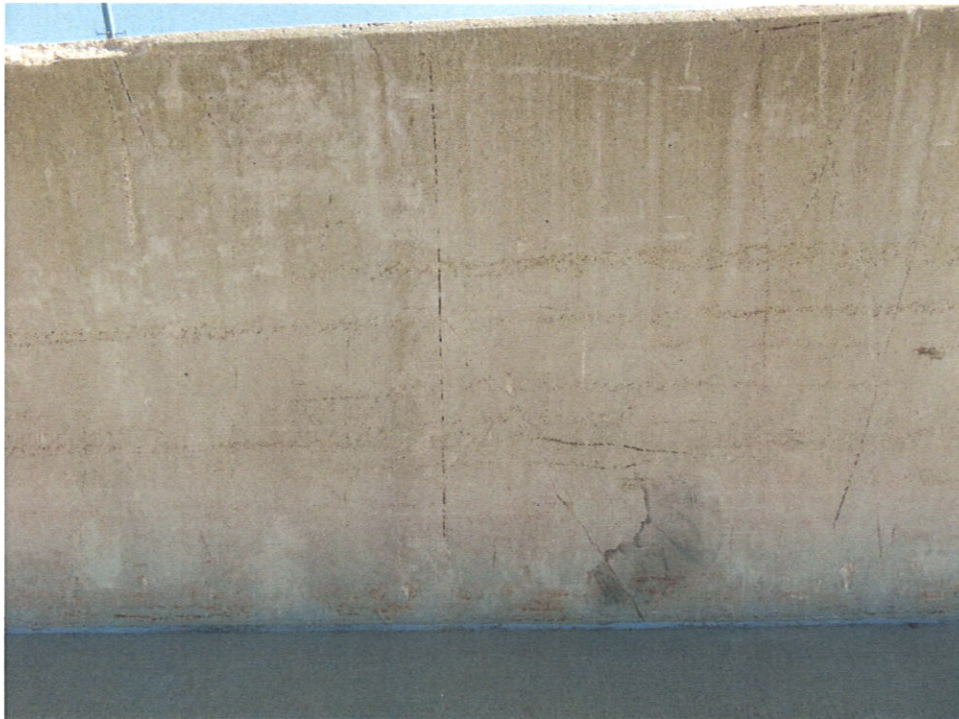
Photo 22 – Example of Diagonal Crack Along East Wall of Rooftop Level
