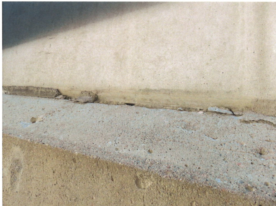
Photo 14 – Deteriorating Grout/Caulk in Horizontal Joint of North Wall of Main Level
