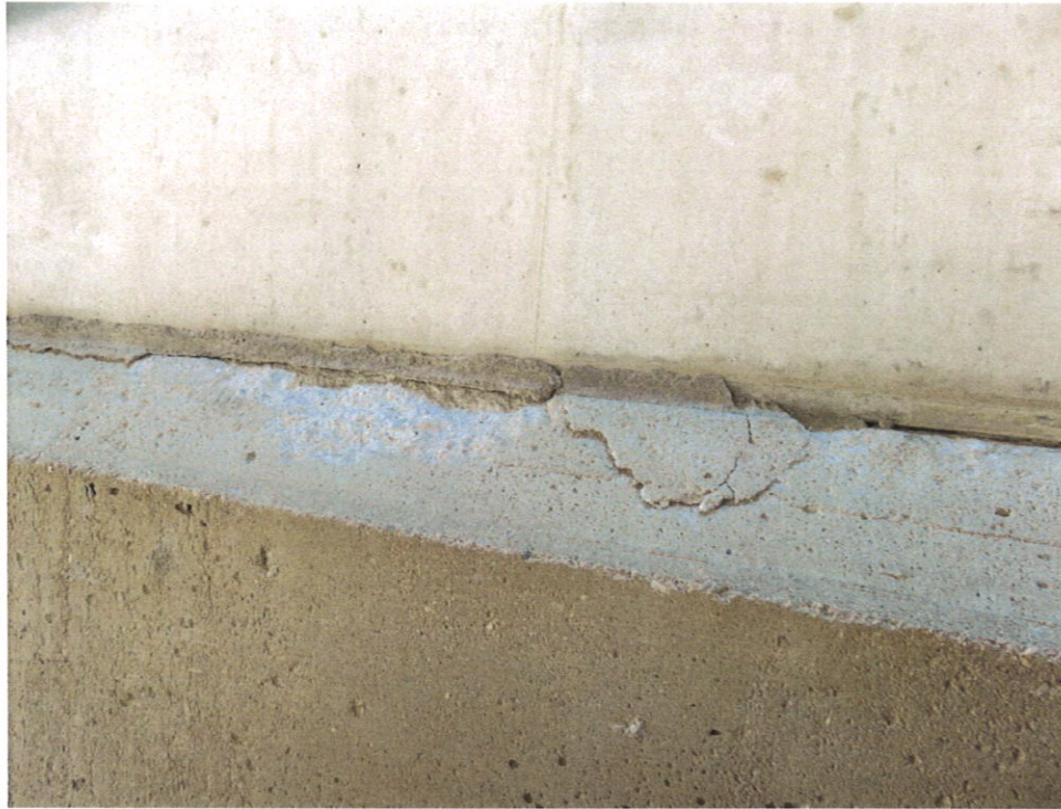
Photo 13 – Spalled Concrete in Horizontal Joint of North Wall of Main Level
