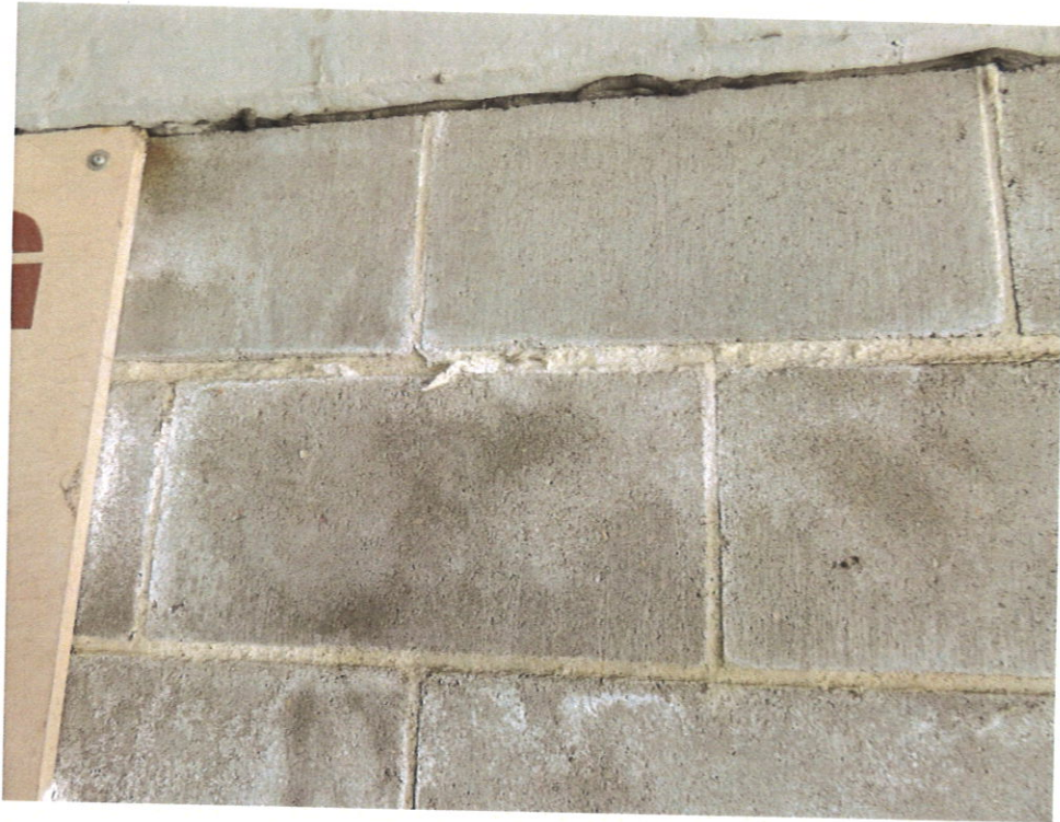
Photo 29 – Evidence of Soft Mortar Joints in CMU on East End of Garage
