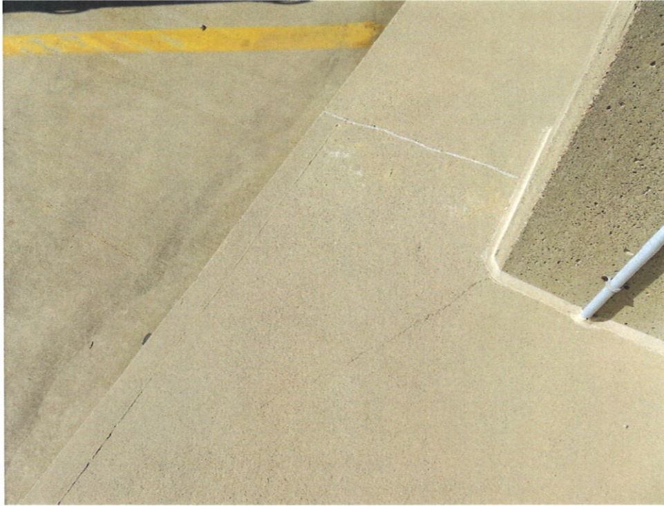
Photo 9 – Example of Hairline Cracks in Sidewalk on North Side of Rooftop Level
