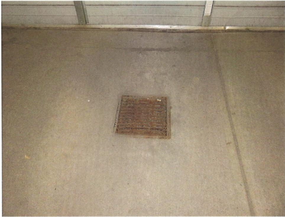
Photo 17 – Floor Drain Clogged with Dirt & Debris Near Overhead Door on East End of Lower Level
