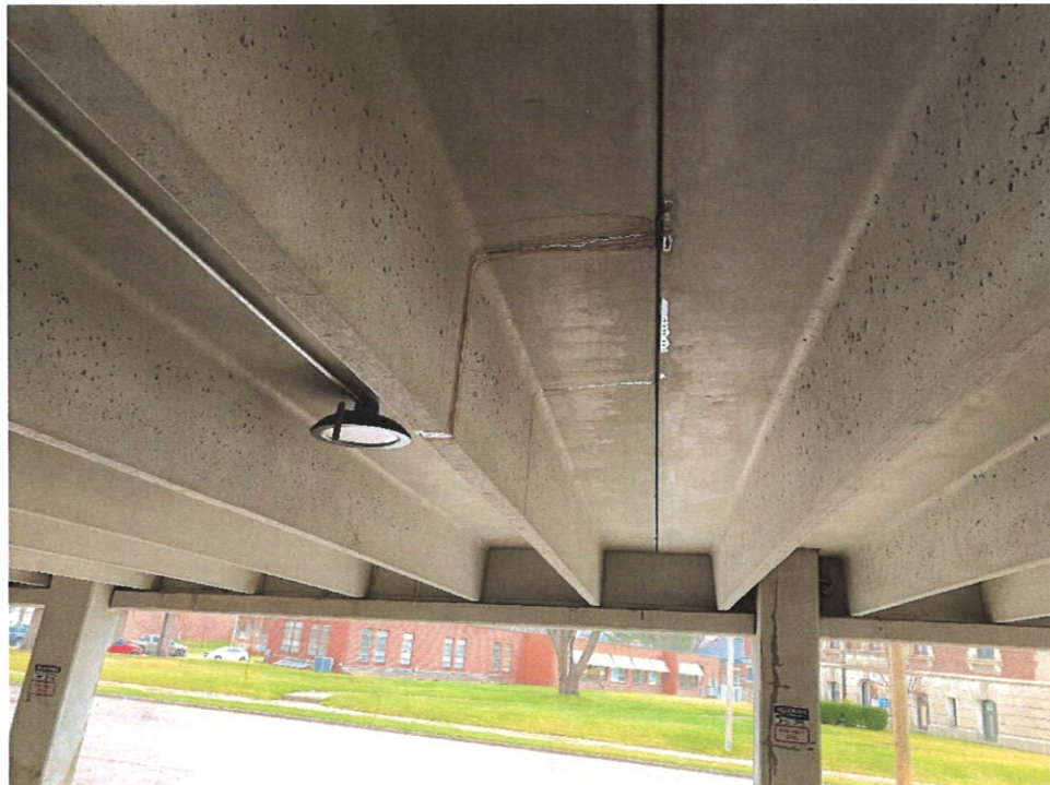
Photo 8 – Example of Rainfall Leak from Rooftop Level
