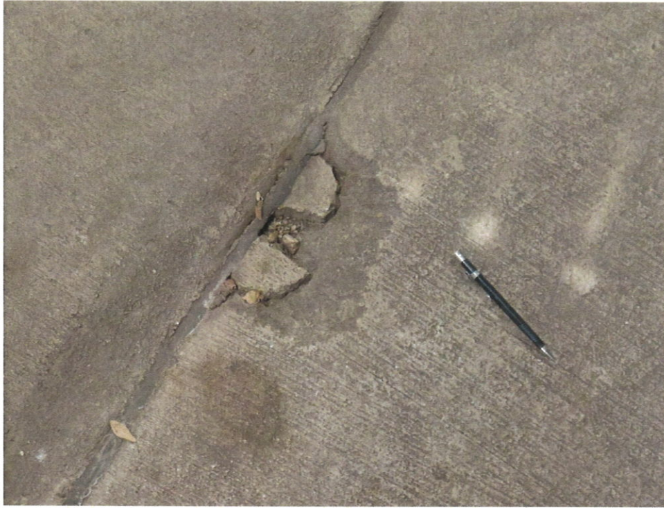
Photo 15 – Example of Spalled Concrete Along Joint Edge in Lower Level
