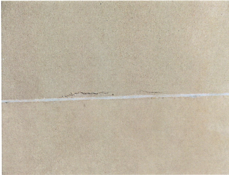
Photo 5 – Example of Spalled Concrete on Rooftop Level
