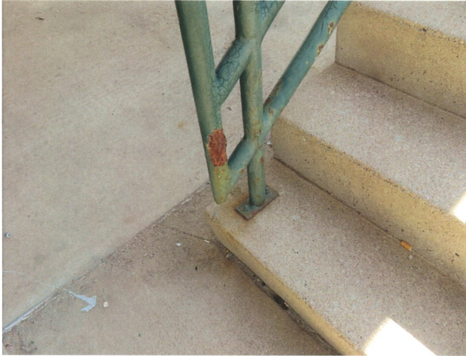
Photo 21 – Example of Rusted Surface of Railing in Northwest Corner of Garage
