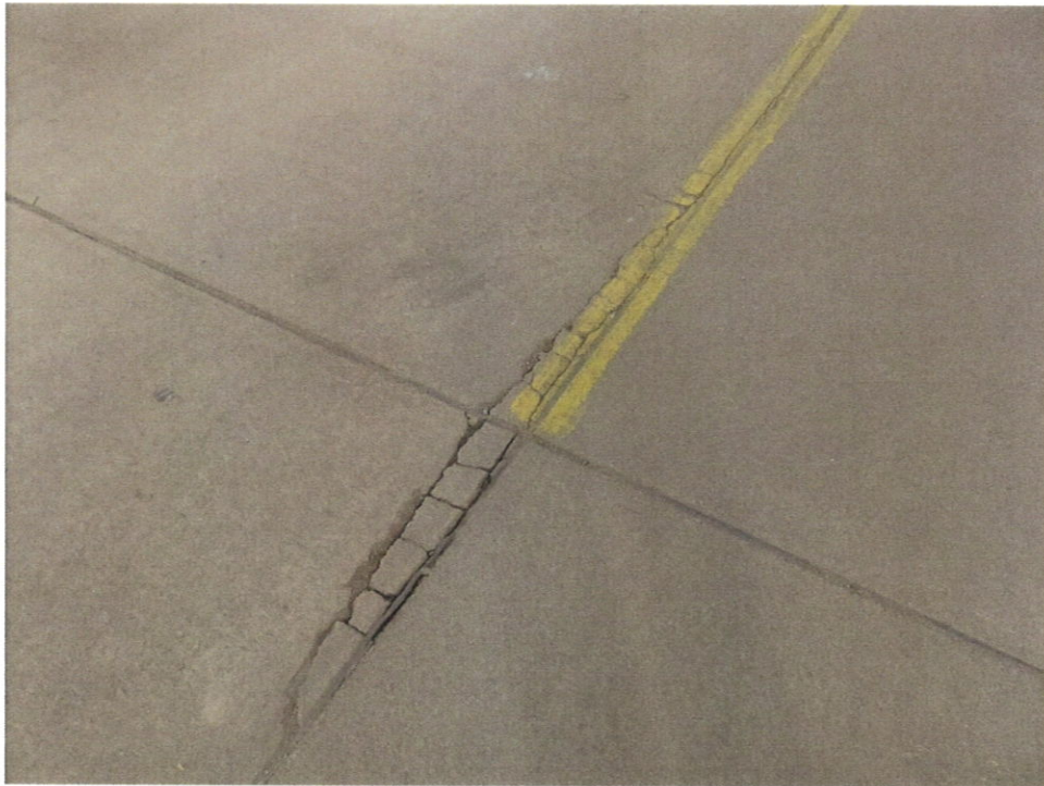
Photo 16 – Example of Spalled Concrete Along Joint Edge in Lower Level
