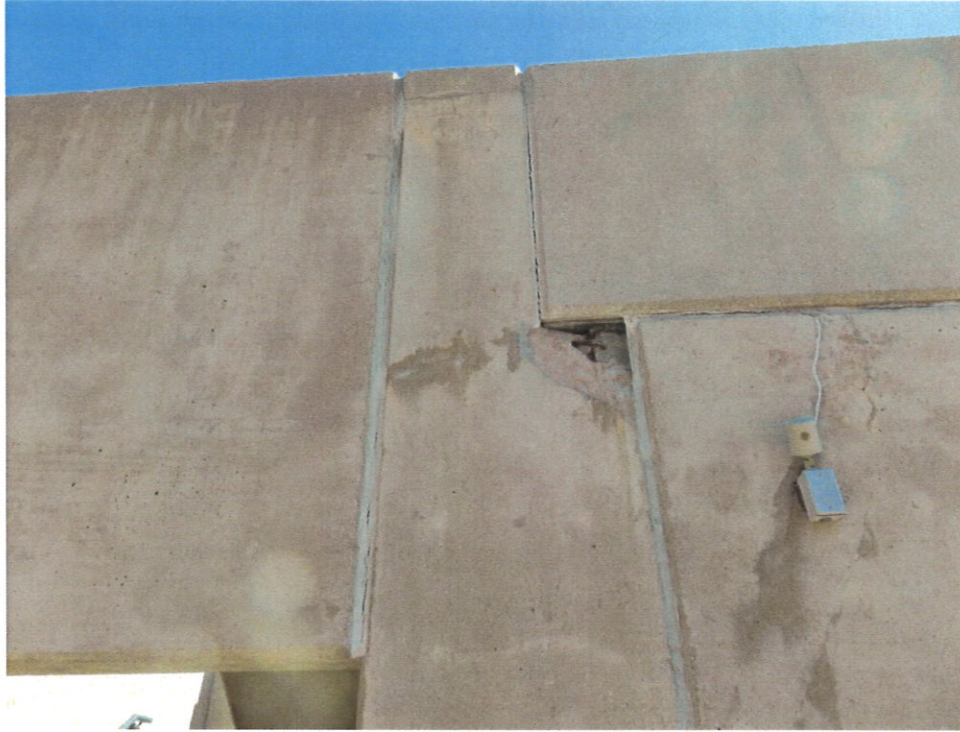
Photo 25 – Spalled Corner of Exterior Precast Column on West Face of Garage
