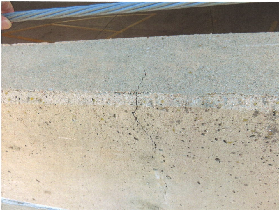
Photo 24 – Vertical Crack Along Interior South Wall of Northern Half of Rooftop Level
