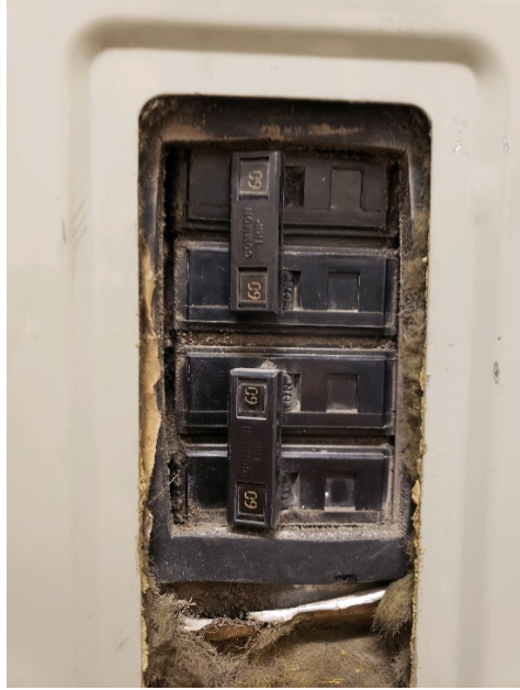
Furnace and Condenser 1. (larger unit west wing) See RFQ section 200.01 for circuit breaker table.
