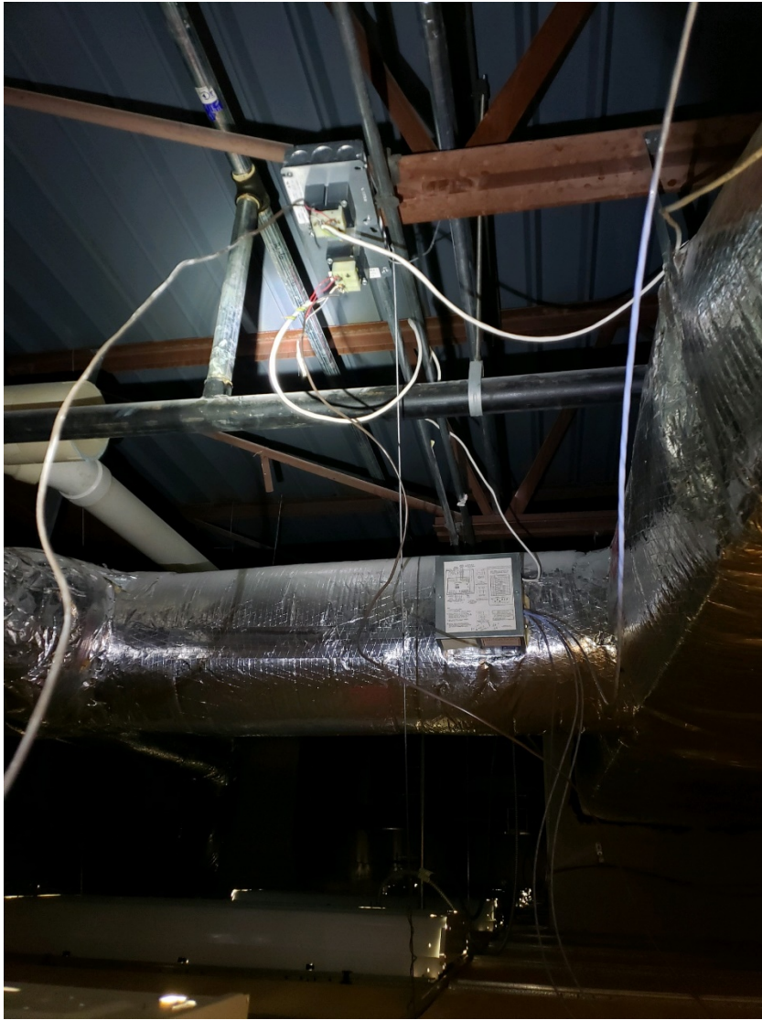
Zone damper control set up.
