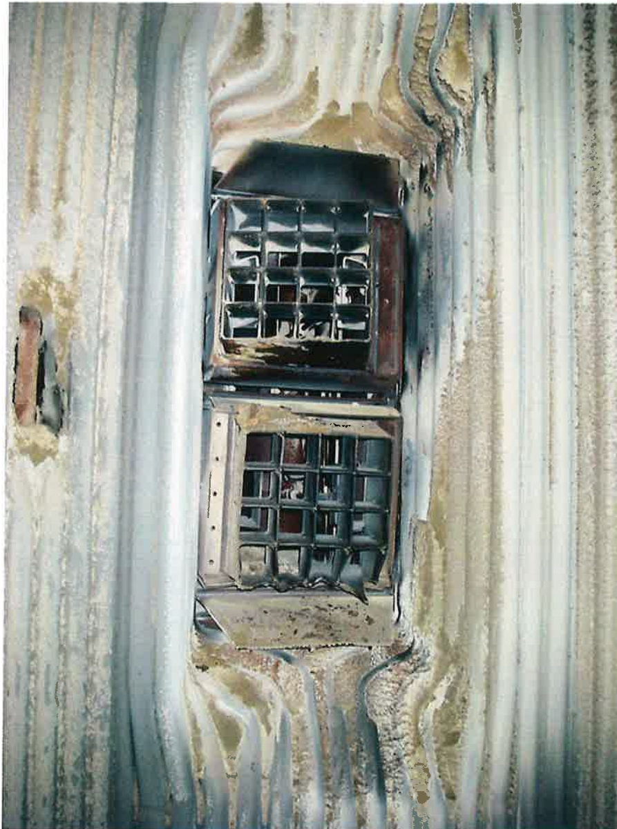
PHOTO #28 Corner 2, separated over fire air nozzles.
