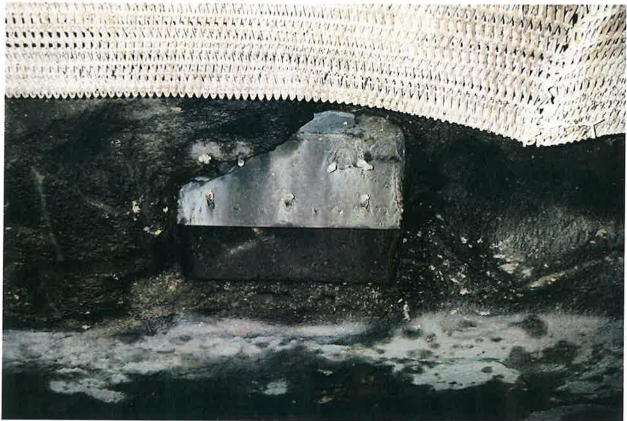
PHOTO #18 Damaged refractory around vacuum breaker.
