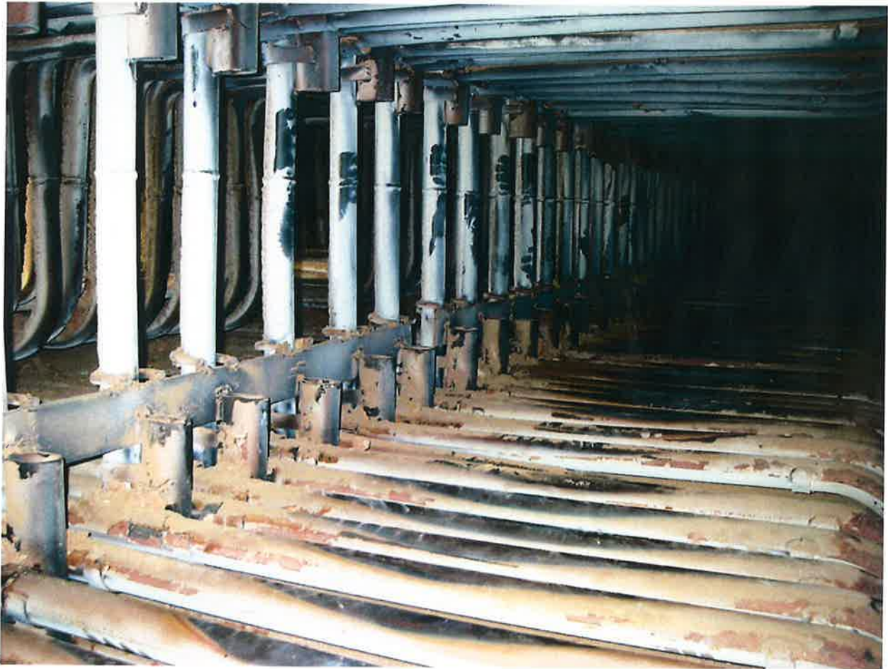
PHOTO #8 Horizontal Superheat tubes between the two banks of tubes.
