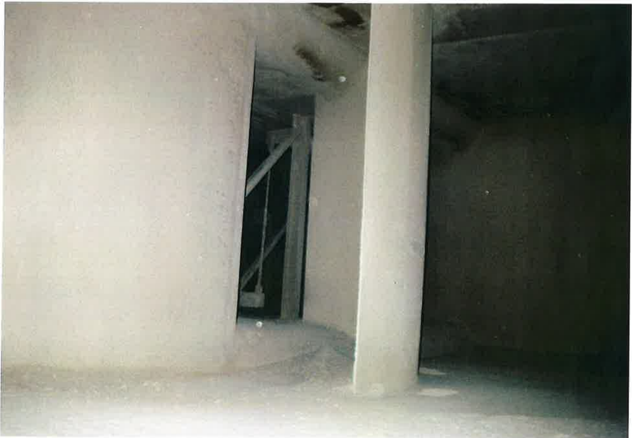
PHOTO #20 Secondary air ductwork, between the air preheater and the left side windbox.
