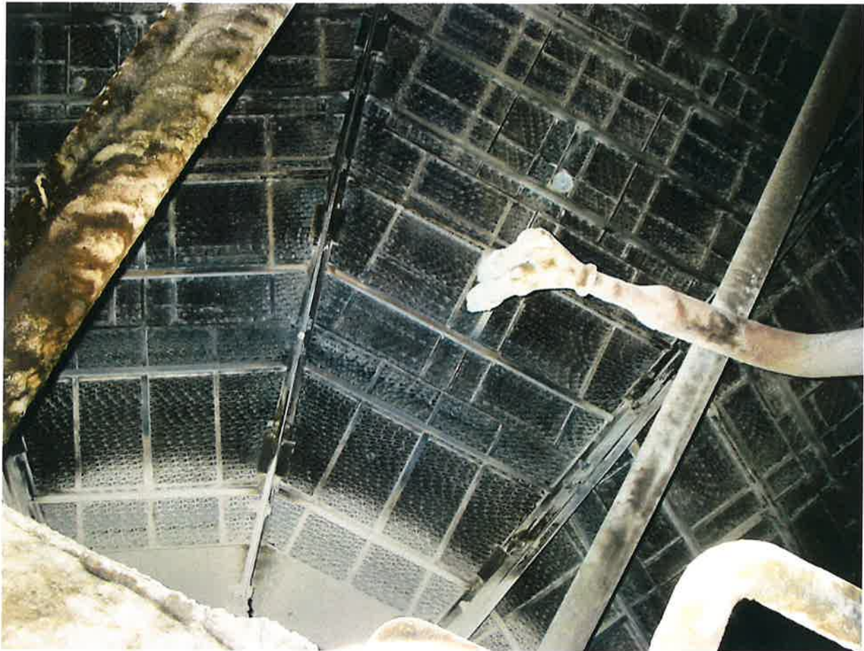
PHOTO #24 Cold end basket elements in the air preheater.
