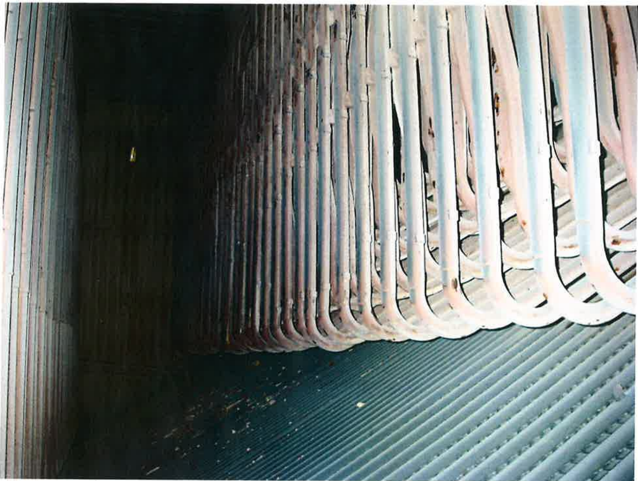
PHOTO #13 Reheat assemblies.
