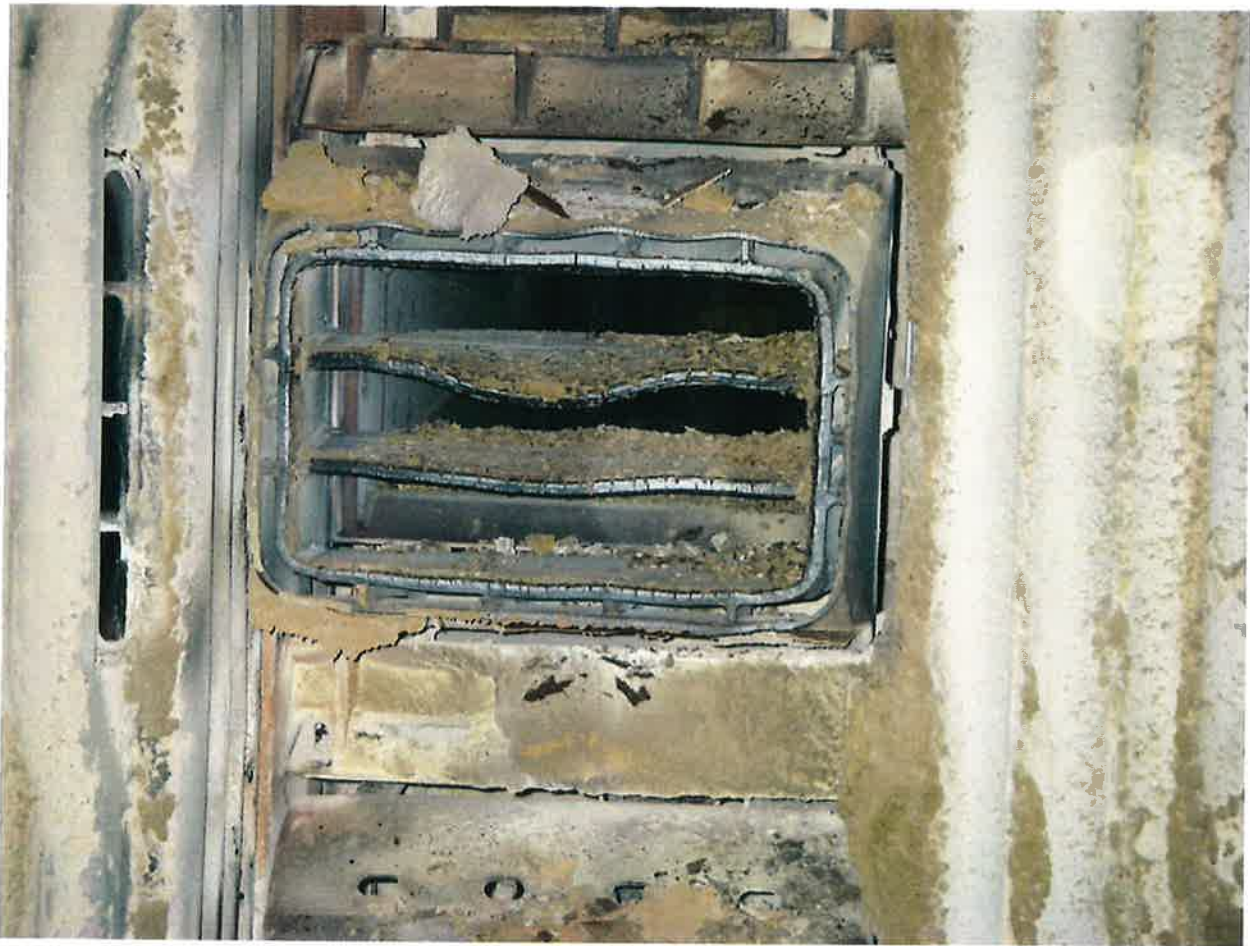
PHOTO #36 Warped and cracked splitter plate in coal nozzle A, corner 4.
