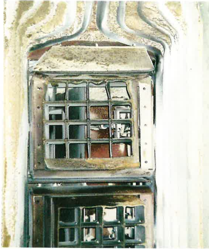
PHOTO #34 Corner 4, separated over fire air nozzles.
