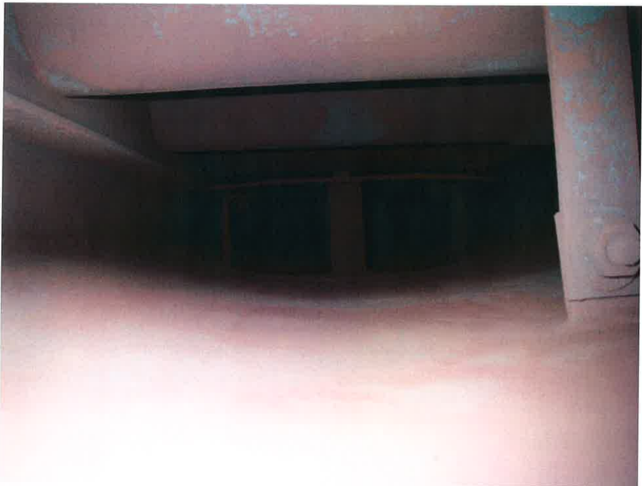
PHOTO #4 Steam drum down comer penetration.
