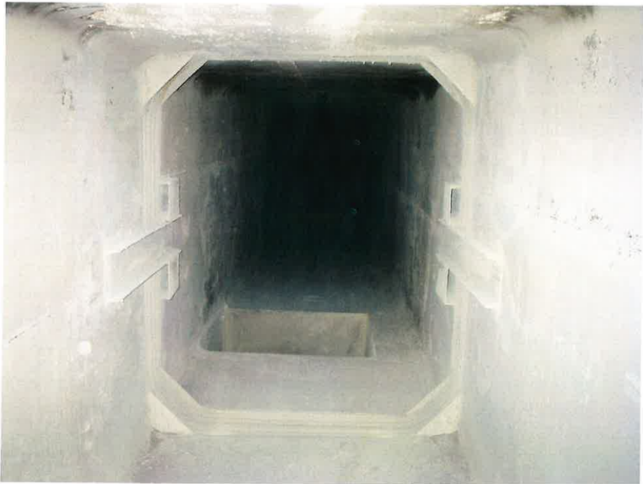
PHOTO #21 Mill hot air duct, with outlets to each coal mill.
