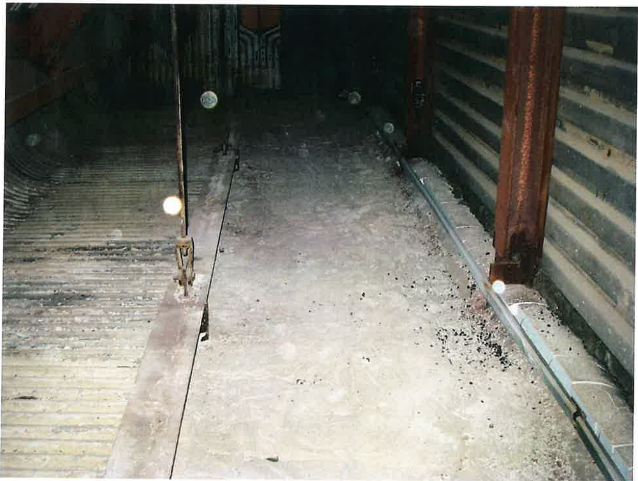
PHOTO #17 Lower dead air space.
