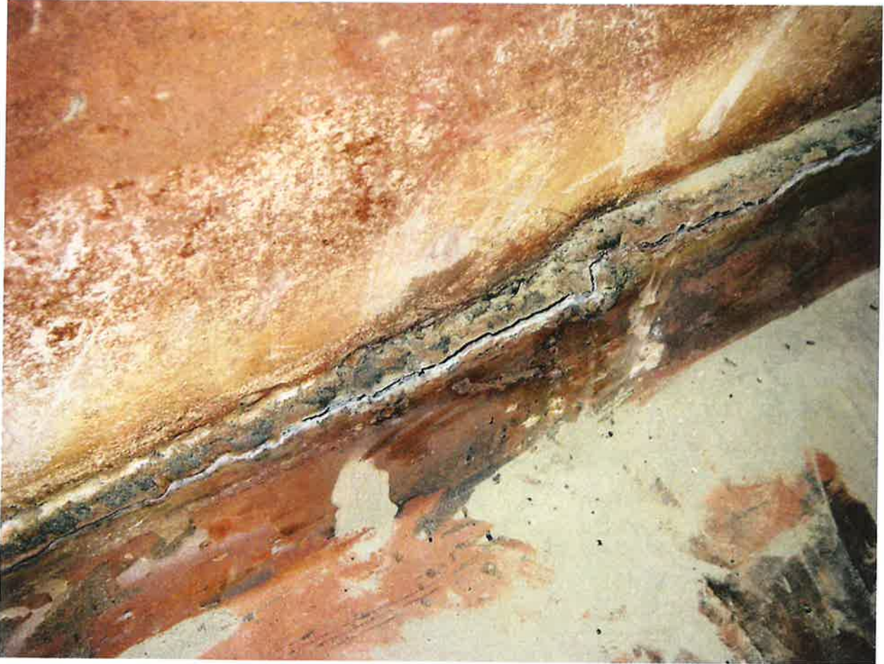
PHOTO #15 Typical penthouse casing crack.
