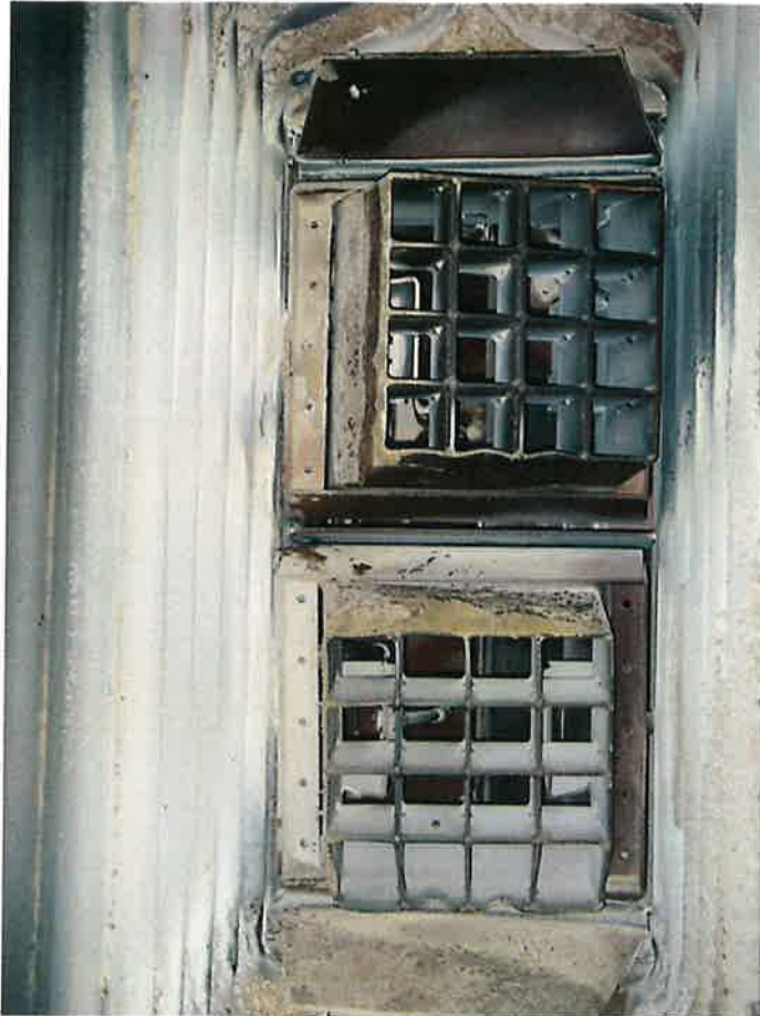
PHOTO #31 Corner 3, separated over fire air nozzles.
