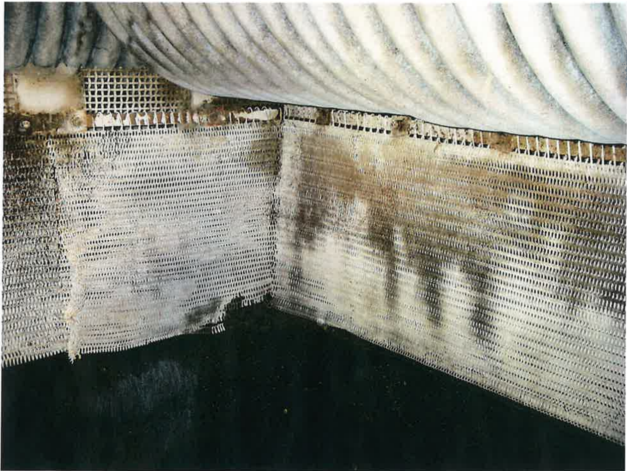
PHOTO #19 Bottom ash drip screens.
