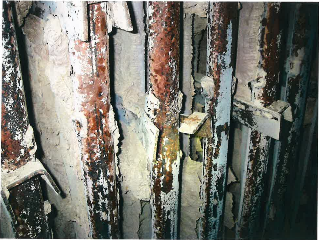
PHOTO #12 Finishing superheater with broken alignment bands.
