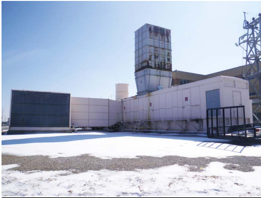
Figure 1 Burdick Station GT1 Combustion Turbine
