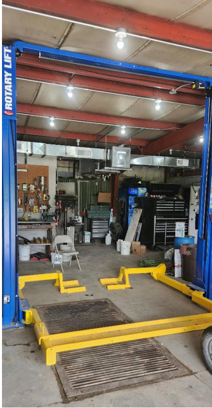
New Shop Lift Installed
