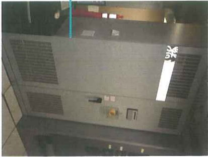
Mark V Control System Cabinet
