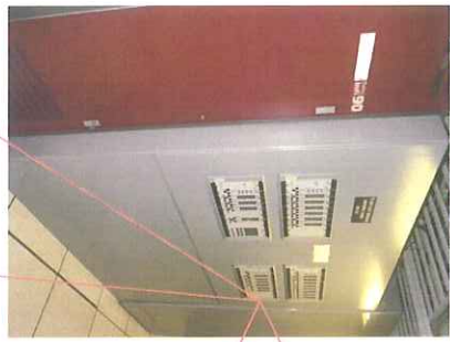
Bently Nevada 3300 System Cabinet
