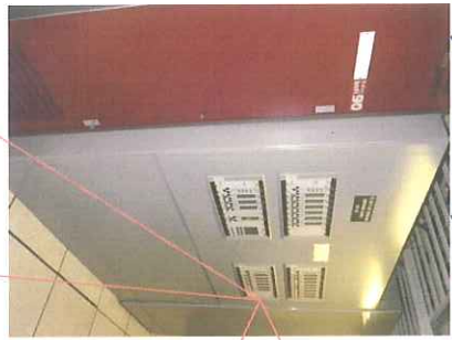
Bently Nevada 3300 System Cabinet
