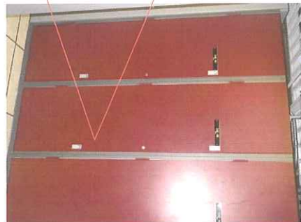
Bailey Infi-90 DCS Cabinets
