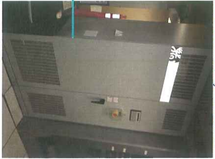
Mark V Control System Cabinet
