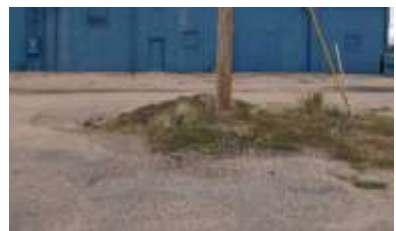
Parking/drive area with deteriorating asphalt and gravel
